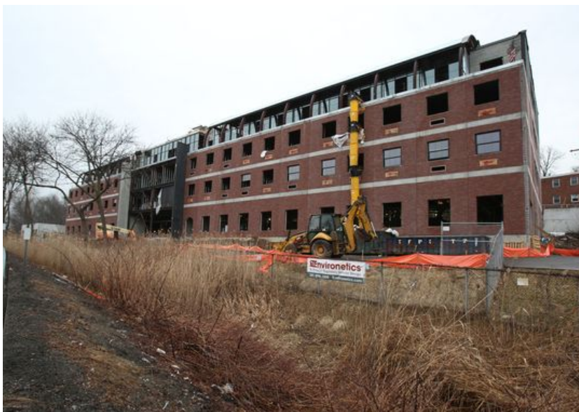
Construction continues at the NYLO Nyack hotel. Rockland County has a hotel tax; local municipalities there do not. (Photo: Peter Carr/The Journal News)
